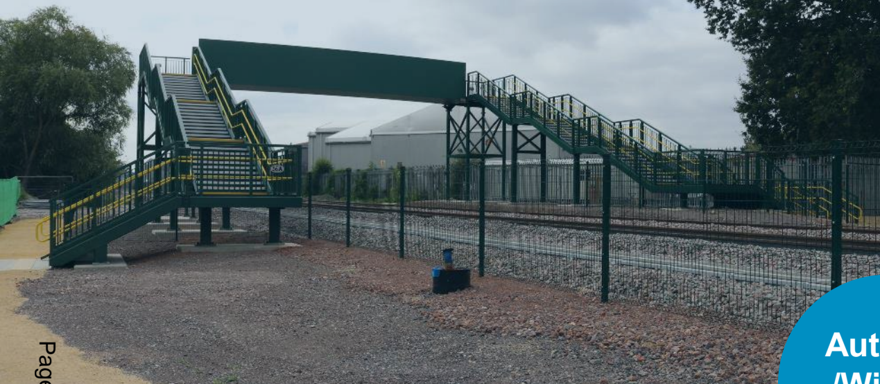
OXD36A Jarvis Lane Footbridge handover – first of five new footbridges to be completed – September 2021
